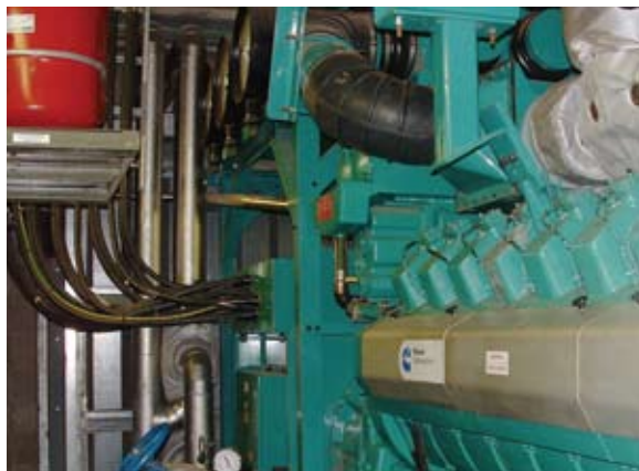
Figure 3: The power plant consists of four 1,370 kVA GQMA low-Btu generator sets, PowerCommand Digital Master Control, low-voltage switchgear and heat exchangers from Cummins Power Generation.
