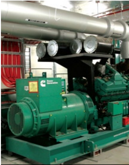
Cummins has installed the standby power system at the hospital, incorporating three 2250 kVA Cummins diesel generator sets.
