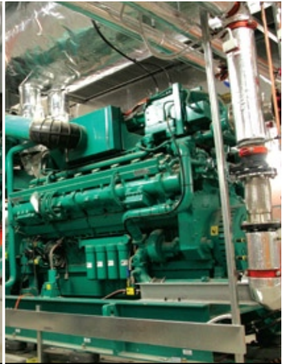
Tri-generation plant at the new hospital features Cummins lean-burn gas generator sets.
