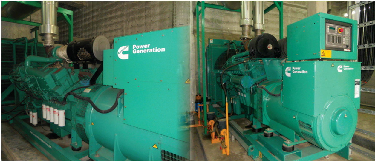
Operations continue on with the support of fully integrated power system comprising of (Left) C1400D 5/KTA50G3 (1250 kVA), and (Right) C700D 5/TA28G5 (640 kVA)
