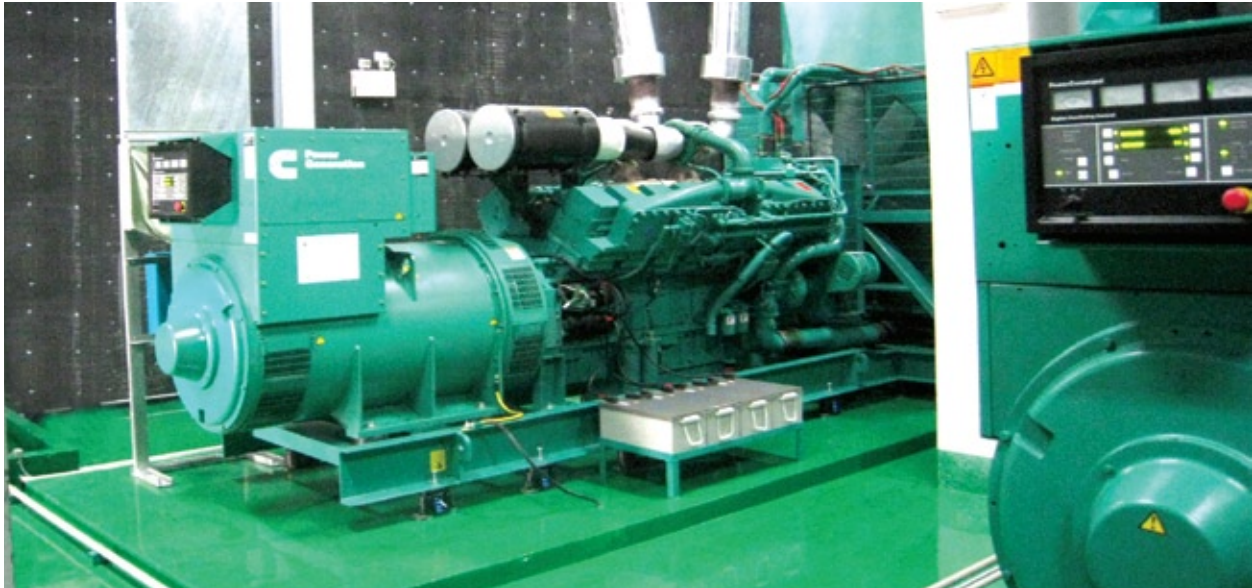
Two units of C1675 D5A with DMC1000 were integrated with an existing 1120 DFCL to provide the electrical backbone for the Srinakarini operations network.
