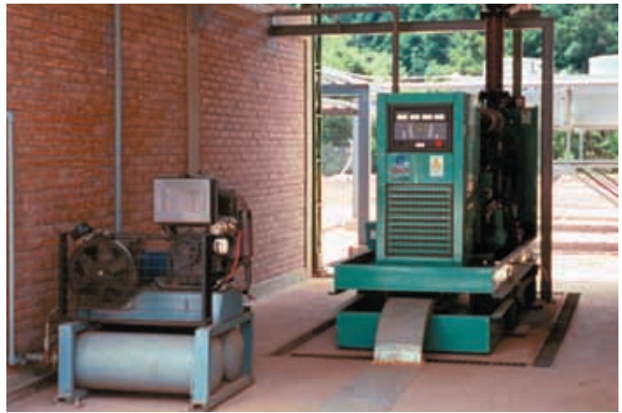
A Cummins Power Generation 275 kW diesel generator provides emergency backup and "black start" capability at the San Alberto gas field facilities.
