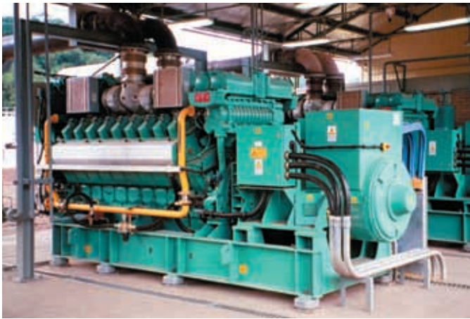
Two 1.25 MW lean-burn gas generator sets from Cummins Power Generation provide all the power for the San Alberto gas processing plant that feeds the Bolivia-Brazil pipeline.
