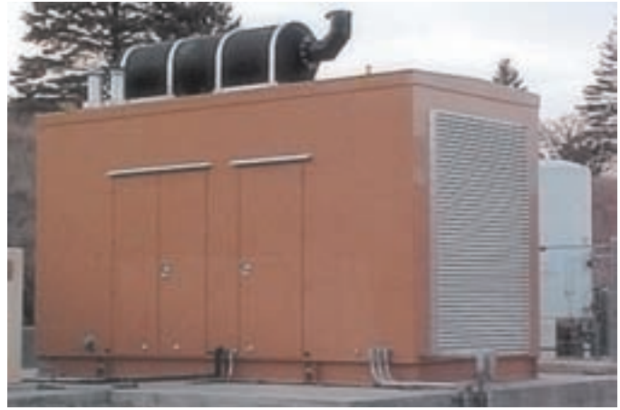
The 600 kW generator is housed in a 20' x 10' weatherproof container on the hospital grounds.
