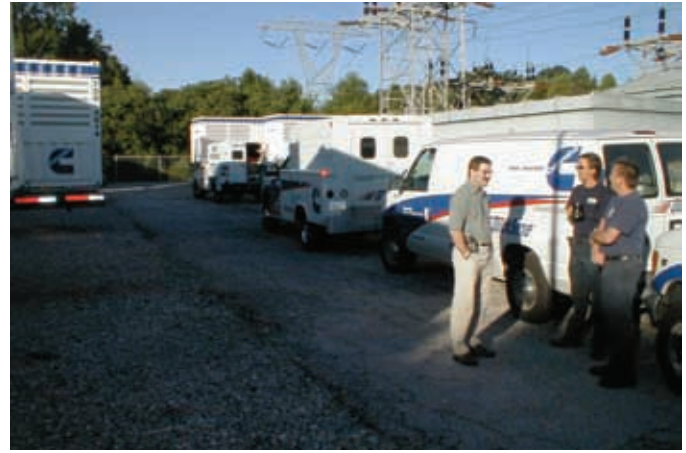
First Energy Corporation and Cummins Power Generation worked together to use on-site Rental Power units for cost-efficient peaking power.
