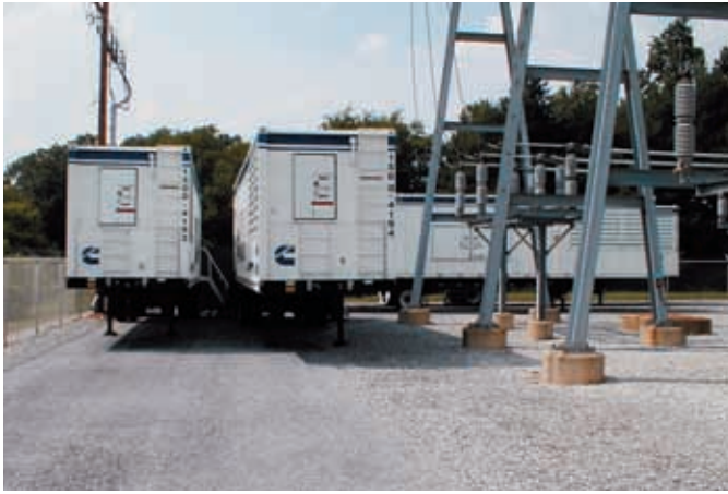
Rental Power units from Cummins Power Generation, ranging from 750 kW to 2 MW, fit easily in substations.
