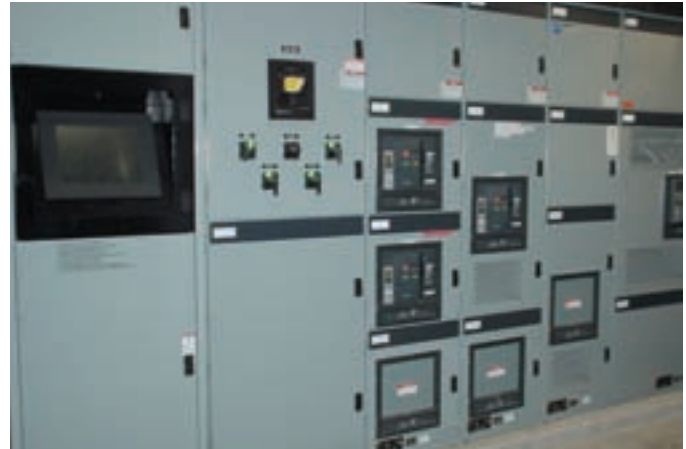
PowerCommand digital controls provide redundancy and real-time information in a smaller footprint; this installation occupies 25 percent less space in the mechanical room than analog technology.
