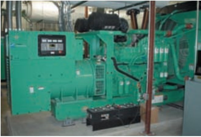
Two 1 MW Cummins Power Generation units occupy less space than the three lower-capacity units they replaced.
