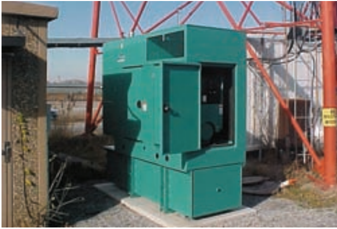
During a utility outage, the Cummins 40 kW diesel generator can power this cellular antenna site for up to three days without refueling.
