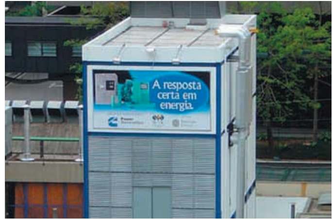
In the city of São Paulo, this compact standby facility contains three low-emissions Cummins Power Generation 1750 kW lean-burn natural gas engine generator sets.
