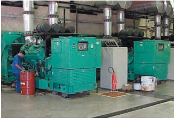
The Anápolis generating station features 33 Cummins Power Generation diesel generating units with a total continuous power rating of 44.3 MW.
