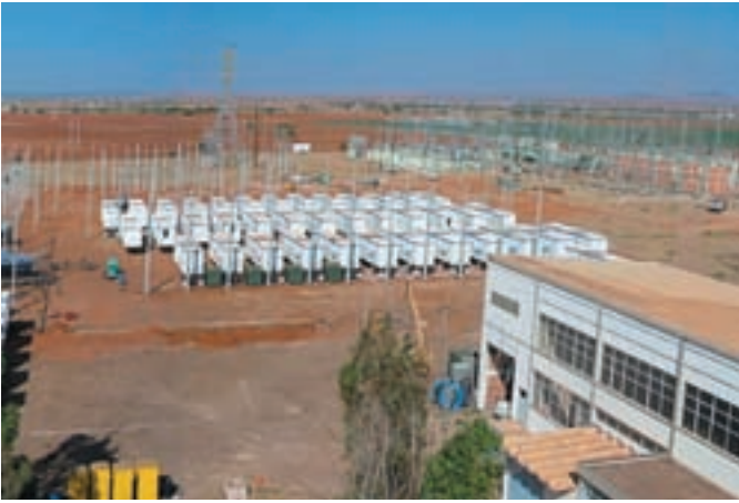
The 170 MW emergency power plant in Zacatecas, Mexico, used the large Cummins Power Generation North American Rental Power fleet.
