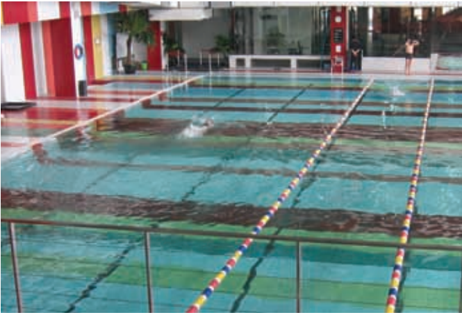
Waste heat from the Cummins Power Generation generator set is used to heat the center's swimming pool and domestic hot water system.
