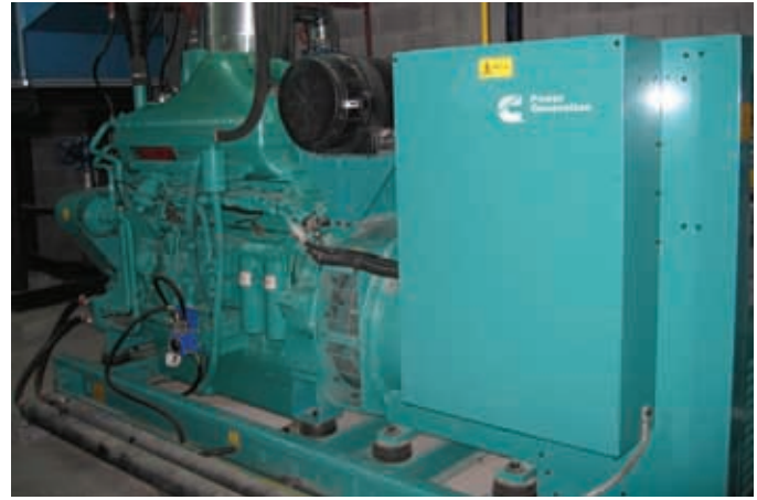
The Cummins Power Generation QSK19G lean-burn natural gas engine generator produces 315 kW of electricity and 1.5 million Btu of heat per hour.
