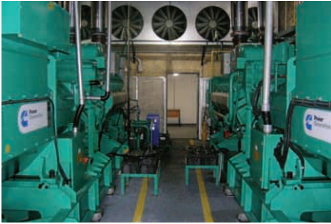
Three gas-powered generator sets are used for peak demand periods and to guarantee power in the event of a utility outage or power crisis.
