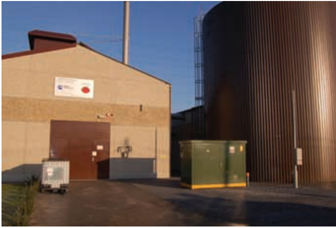
Buffer tanks near the power building store hot water that is released at night to warm the greenhouses.
