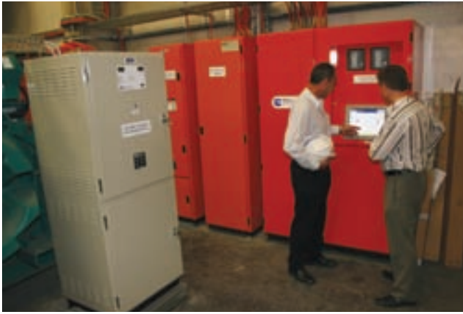
Three new Cummins Power Generation diesel generator sets plus PowerCommand digital paralleling equipment provide standby power and control for the Queensland Cultural Center.
