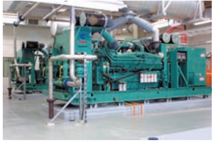
The standby system from Cummins Power Generation includes one 350 kW and two 1500 kW generator sets.
