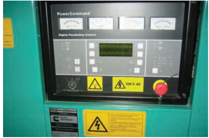
The PowerCommand digital master control assures a smooth transition from utility to generator power.
