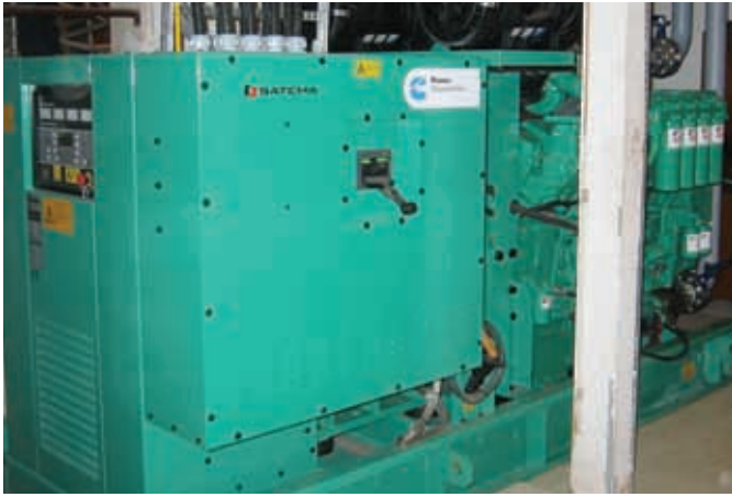
A new 819 kVA (713 kW) standby generator from Cummins Power Generation supplies the hospital's newest addition.
