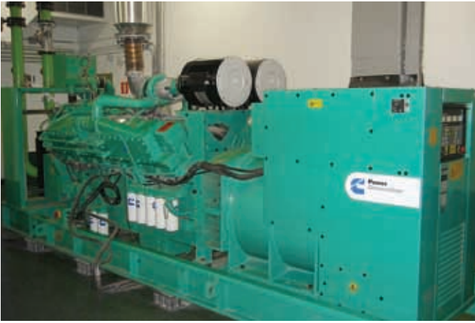
One of two 1.4 MVA C1400D5 generator sets that supply standby power for the El Corte Ingles at Hipercor Xanadu shopping mall.
