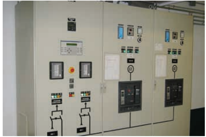
Switchgear from Cummins Power Generation provides critical control during power outages or monthly testing.
