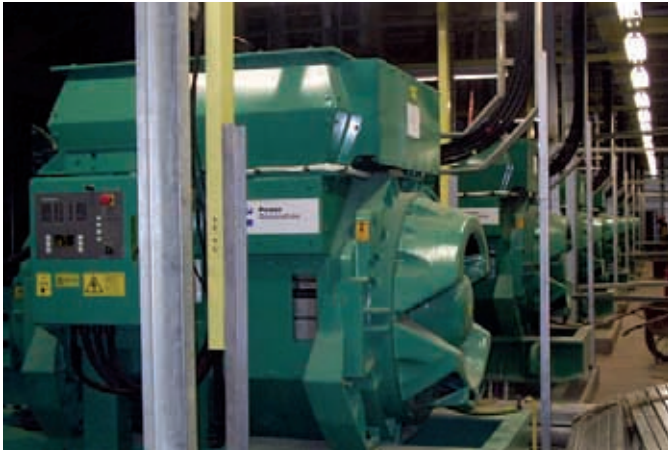
Ten Cummins Power Generation diesel generator sets compose the standby power system that protects IVO's semiconductor production in the event of a utility power failure.
