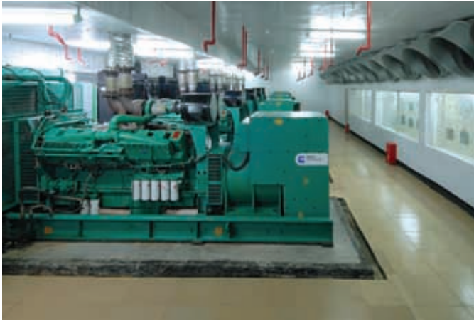
Four Cummins Power Generation generator sets operating in parallel ensure continuous services for hotel guests and allow generator-set maintenance without power interruption.
