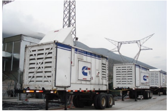
Eleven 1 MW and two 2 MW trailerized Rental Power units provide 15 MW of power to the plant during equipment testing and startup.
