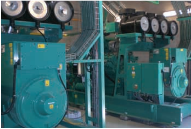
Two Cummins Power Generation natural gas generator sets are the heart of INDITEX Group's cogeneration system in Tordera, Spain.
