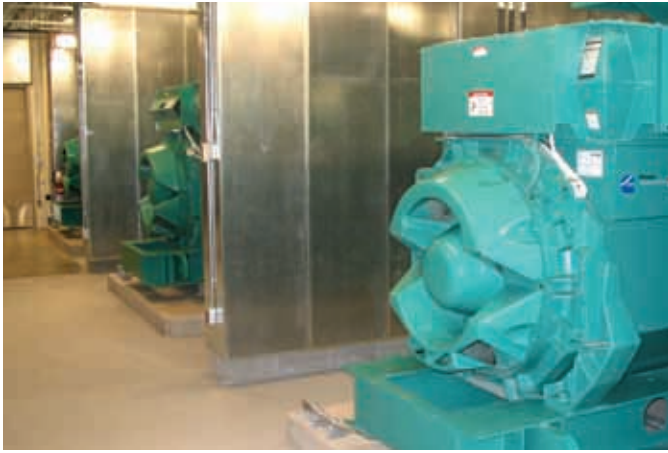
Three 2 MW diesel generator sets from Cummins Power Generation provide standby power for Alberta Children's Hospital.
