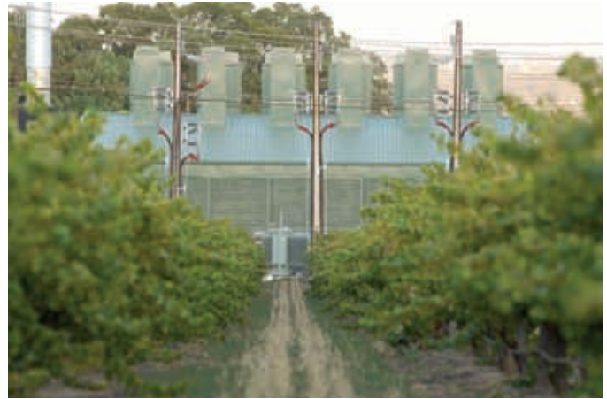
The plant’s 30 QSK60 generator sets from Cummins Power Generation can start up, synchronize and be online providing 50 MW in less than two minutes.
