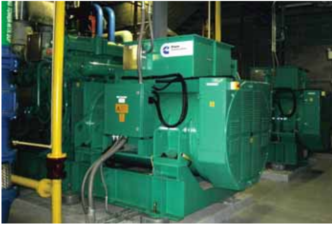
The heart of the cogeneration system is a pair of 1.25 MW gas generator sets from Cummins Power Generation.
