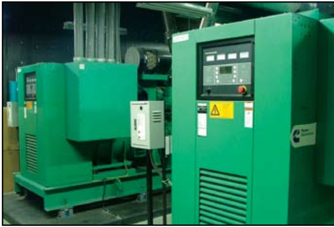
Cummins Power Generation gensets capable of handling high SCR content loads.
