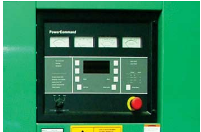
Cummins Power Generation advanced PowerCommand Control ensures quick start up to power 2000 kVA facility load.
