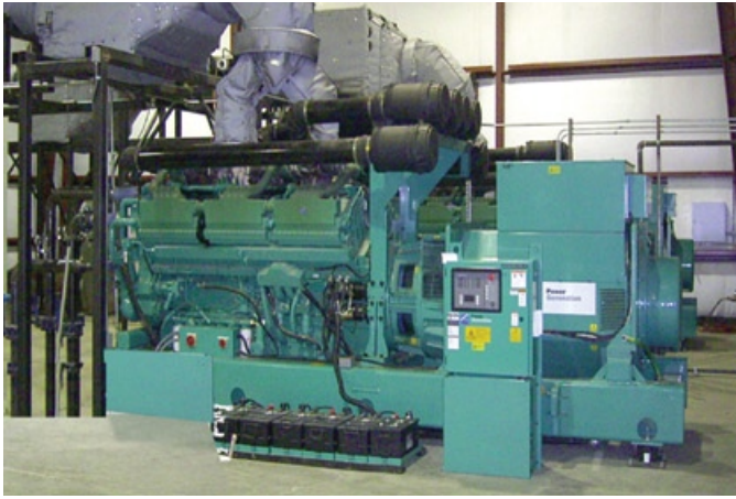
The “micro-grid” system includes six Cummins Power Generation 2 MW prime power diesel generators (model DQLA) powered by 78-liter Cummins engines.
