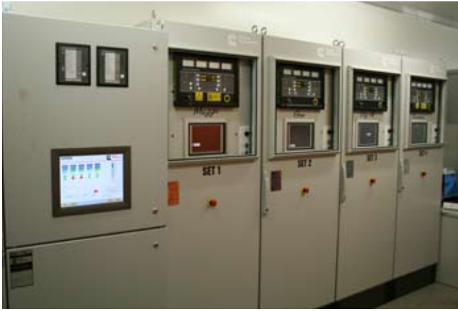
A Cummins Power Generation DMC300 Digital Master Control system is used for load demand management of the complete power station.
