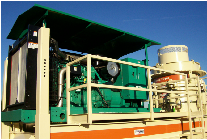
Two Cummins Power Generation diesel generator sets were retrofitted and installed on top of the chassis of two separate crushers.
