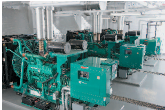
Three 1000 kW generator sets after installation. One is always in reserve. (Photo courtesy of Trumpie Photography.)
