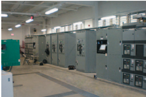
The paralleling switchgear and a generator set being installed at the new data center.
