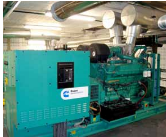
Cummins C825 D5A generator set is installed with a remote cooling system.
