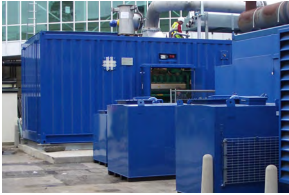
Frimley Park Hospital has taken a huge step toward reducing its carbon footprint with a new tri-generation project featuring a (CHP) plant driven by Cummins Power Generation Inc.
