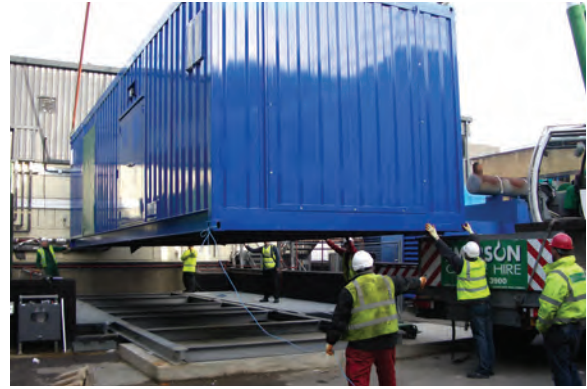
Equipment was delivered in an extremely tight space for maneuvering, requiring close supervision of craning equipment from Cummins Power Generation's delivery team.
