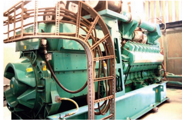
Five C1750 N5C natural gas generator sets were installed to provide 11,000 kVA (8.5 MW) of power.
