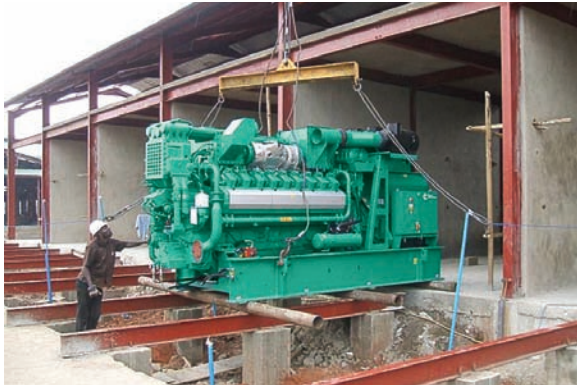
Each generator set was equipped with a QSV91 Cummins engine and Powercommand® control.
