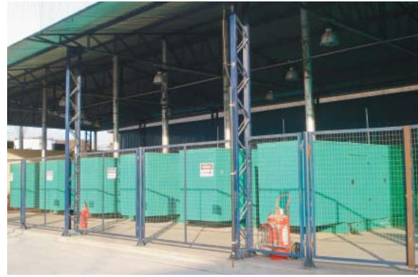
The generator sets installed in sound-attenuating enclosures at the Alubar plant in Barcarena, Brazil.
