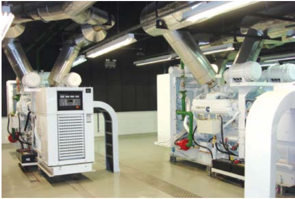
The Cummins Model DFHD generator sets and digital controls installed at Rede Globo.
