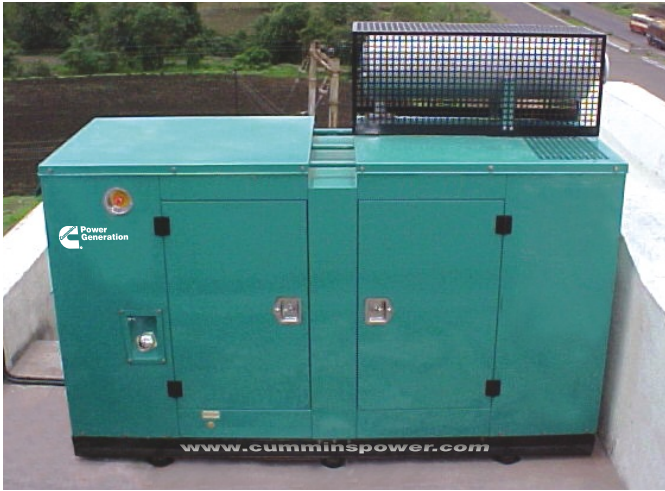
Rooftop installation for IDEA Cellular's cell site
