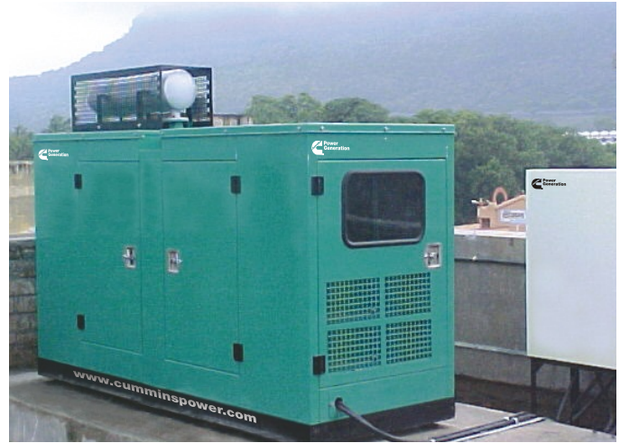
Cummins Power Generation generator set with micro processor based Auto Mains Failure panel
