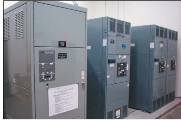
The PowerCommand® Automatic Transfer Switch and other control equipment.
