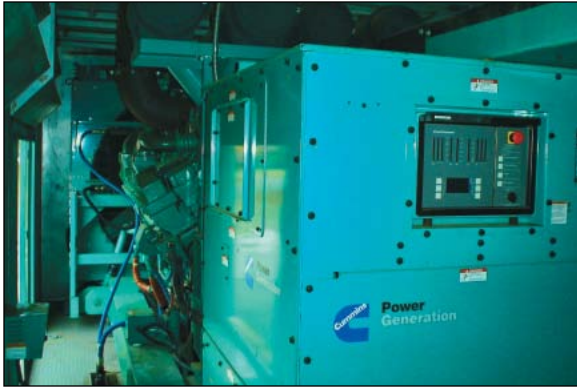
The generator set with control module inside its enclosure.
