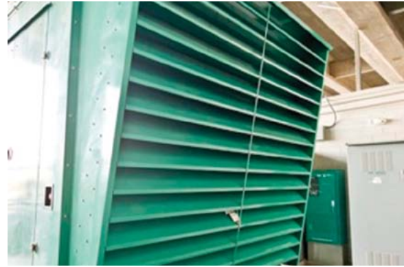
The 800 kW DQFAB generator set and one of the PowerCommand OTPC automatic transfer switches.
