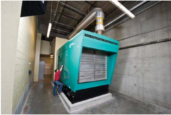
The 1000 kW DQFAD generator set, located near the Target Field loading dock.
