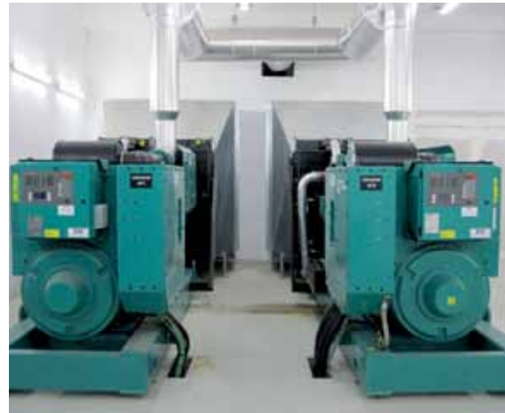
Cummins power solution is housed in a specially designed underground room located in the hospital grounds at a distance from the main buildings to minimise noise and vibration in the hospital.
