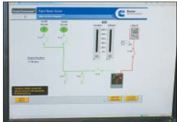
This installation includes a remote monitoring system that allows the maintenance manager to monitor the power system from his desk. A closed-circuit television camera in the generator building makes it possible to read the generator control display from the remote location.
