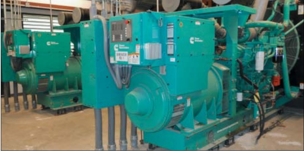
Two 750 kW generator sets serve the factory and the dewatering pumps.
