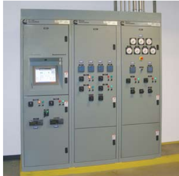
System operation is orchestrated by two PowerCommand® DMC 300 digital master controls and front-accessible switchgear units.
