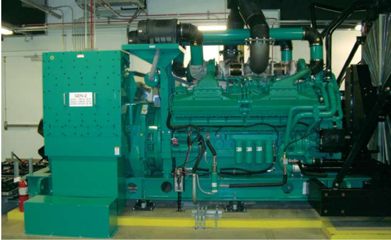
When the second phase is completed, the system will include six 2 MW DQKAB Cummins Power Generation generator sets.
