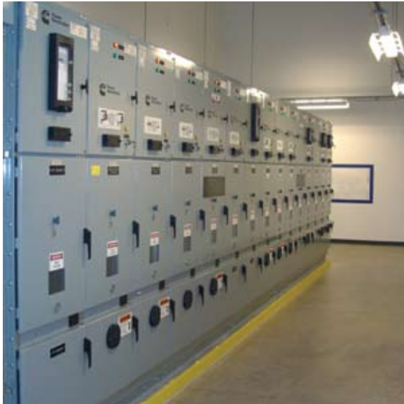
The line of switchgear will provide power transfer between the utility and generator sets.
