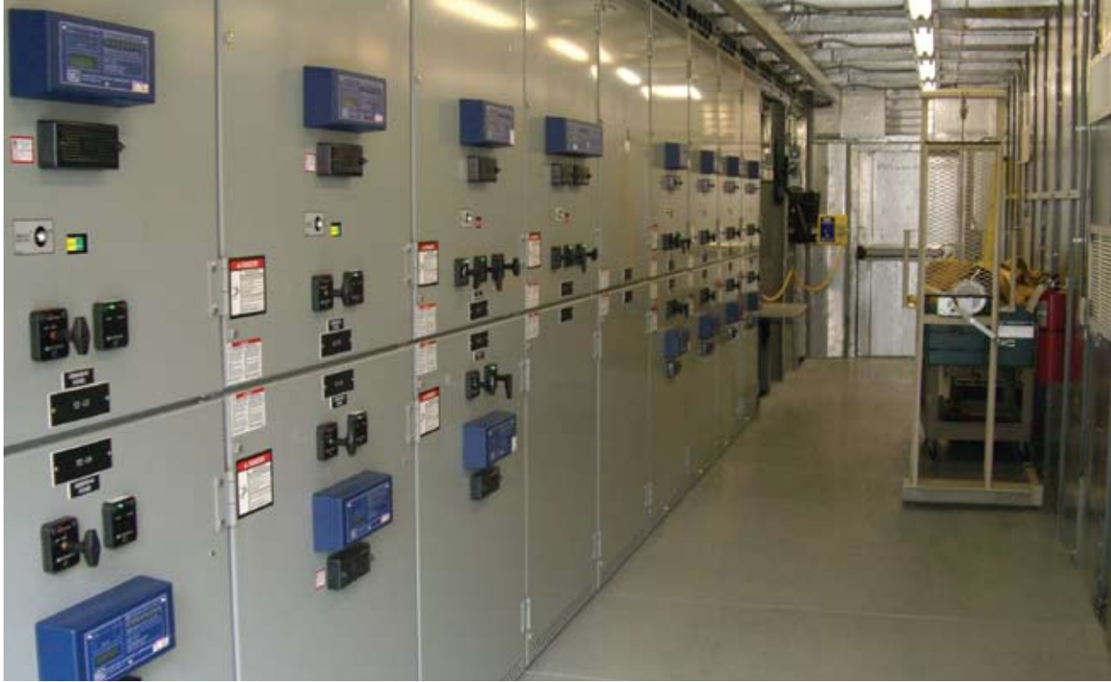
The system provided by Cummins Power Generation includes a PowerCommand® digital paralleling system with a DMC 200 and ten sections of switchgear.
