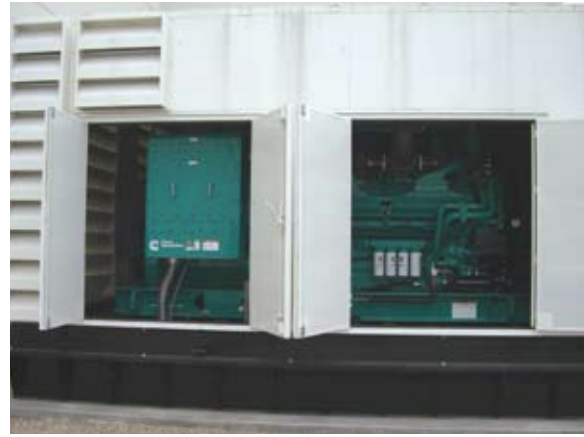
Standby power is provided by two 2 MW DQKAB generator sets in a sound attenuated housing.
