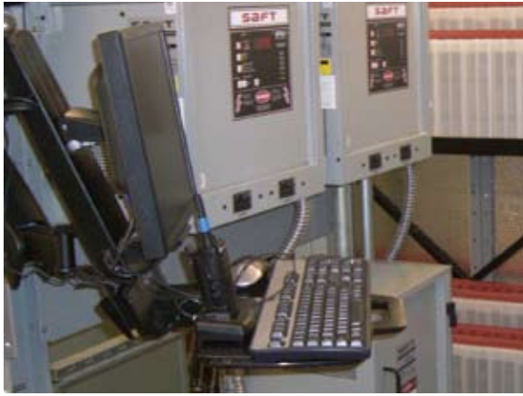
The power system can be controlled from three different locations within the complex.
