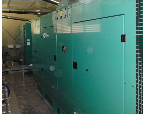
The Cummins power solution comprises two enclosed sets housed in a specially adapted room.
