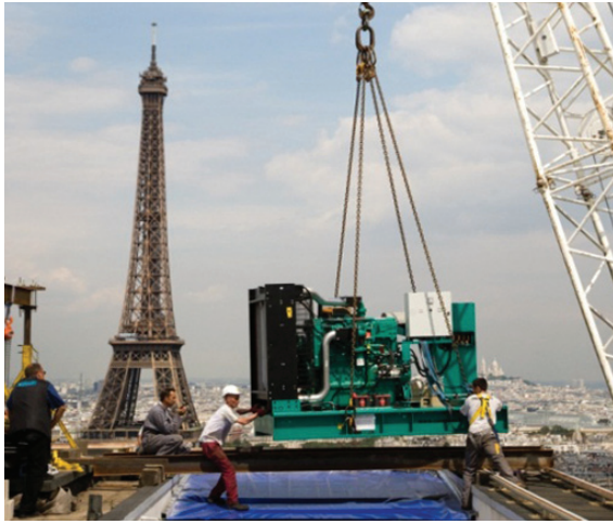
The generator set goes into position on the roof of the Tour Evasion
