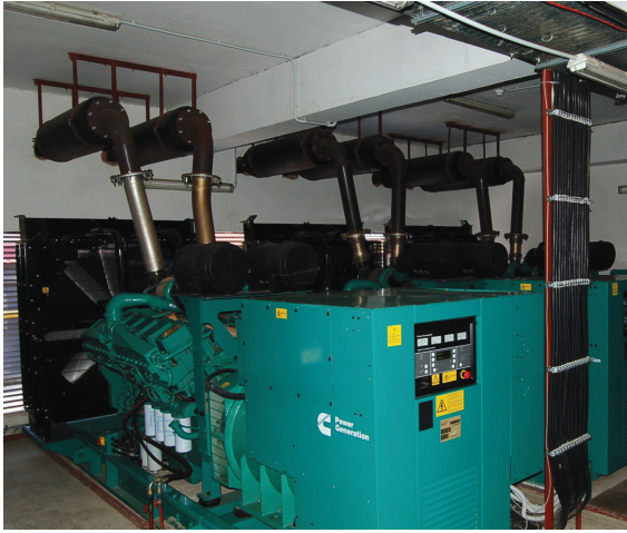
Cummins Power Generation ensures the site is operational 24/7
