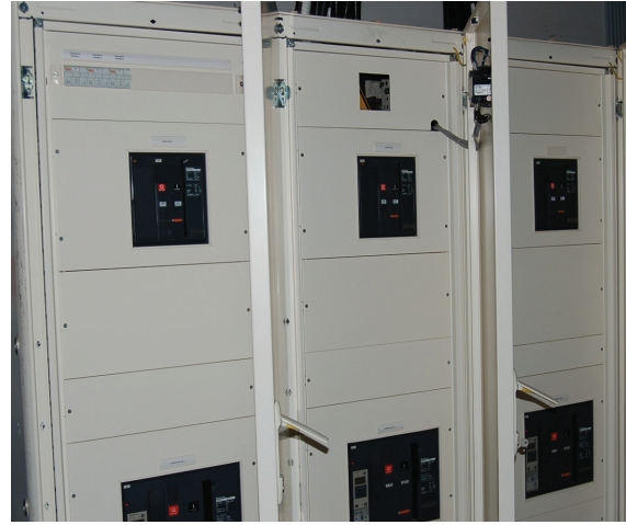
The standby power solution incorporates a PowerCommand® PCC 3100 paralleling system
