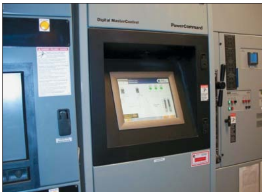
The DMC provides system-level functions, including load add and load shed sequencing, load demand, and system operator interface.
