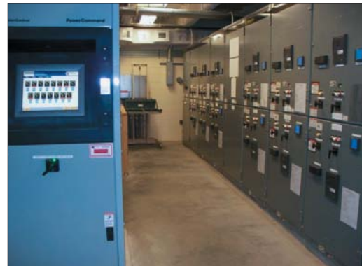
The PowerCommand® DMC with paralleling gear.
