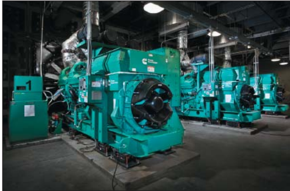
The PowerCommand® generator sets and control equipment installed in the basement of AnMed Health Medical Center.
