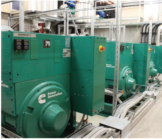
AKSA Würenlos installed three C1675 D5 generator sets
