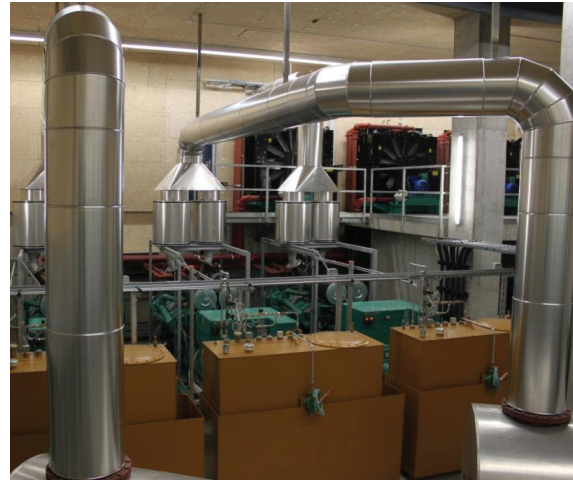
The generator sets are located in a specially designed room
