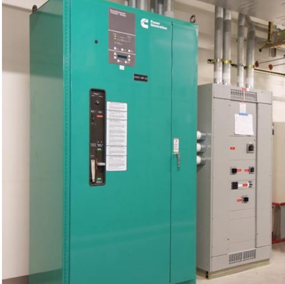
The system includes nine bypass transfer switches: four 2000 amp BTPCs, four 800 amp BTPCs and one 400 amp BTPC.
