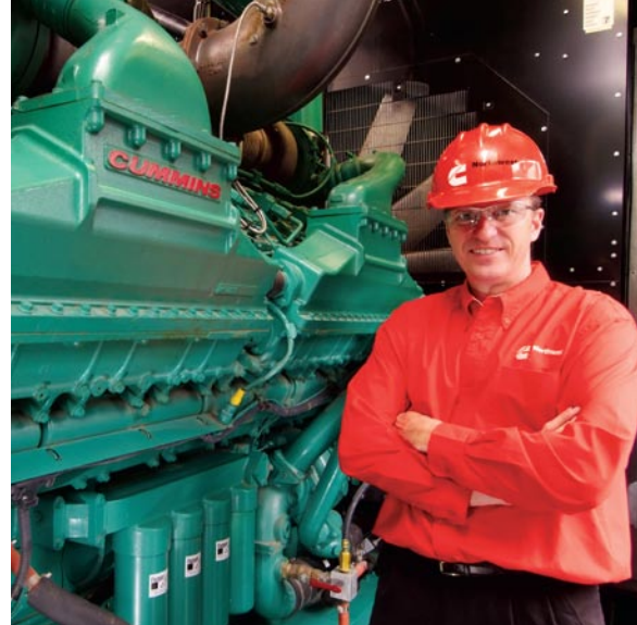
The system is powered by two 2 MW DQKAB generator sets in sound-attenuated housing from Cummins according to Jim Stalnakar, Power Generation sales manager, Cummins Northwest, LLC.
