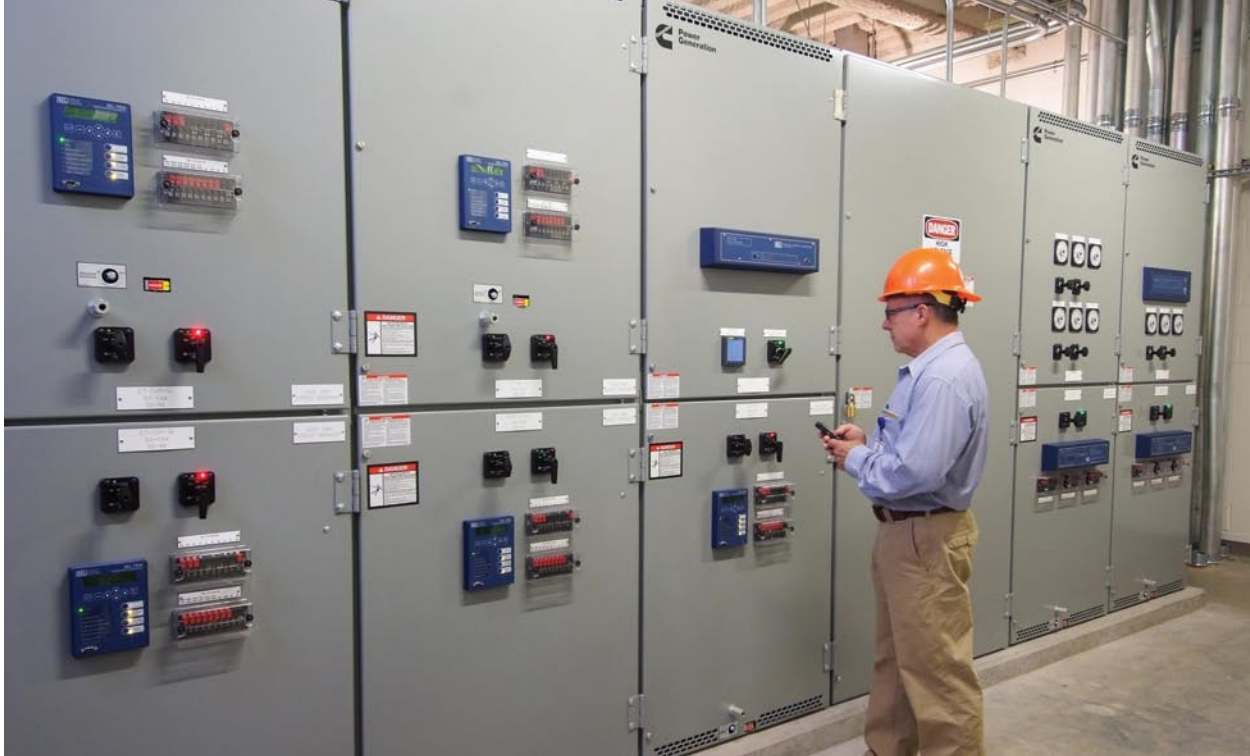
John Hamilton, operations director, Oregon State Hospital, started the project with a series of collaborative discussions with Oregon State Hospital, PGE and AEI. The 4 MW system from Cummins Power Generation included one DMC 300 Digital Master Control and paralleling switchgear.
