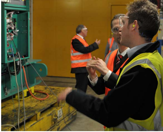
The generator set was put through its paces and performed above the target standard
