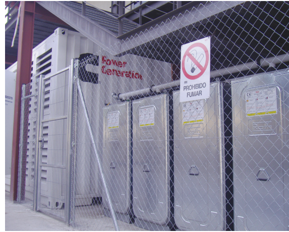
Cummins is providing standby power for the entire hospital site
