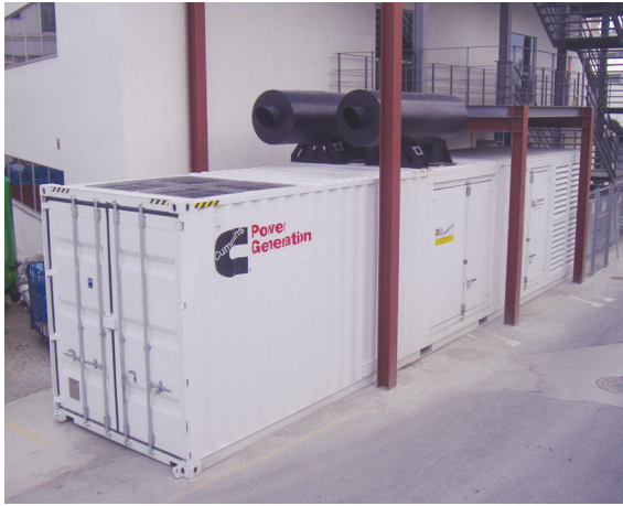
The C2250 D5 generator set is housed inside a 40ft container
